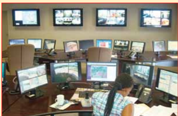
A housing complex control room
